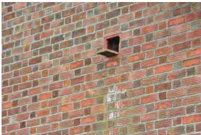
An air brick was opened up to give access for an internal nest box in Pidley Pumping Station at Warboys, Pidley & Somersham IDB.
