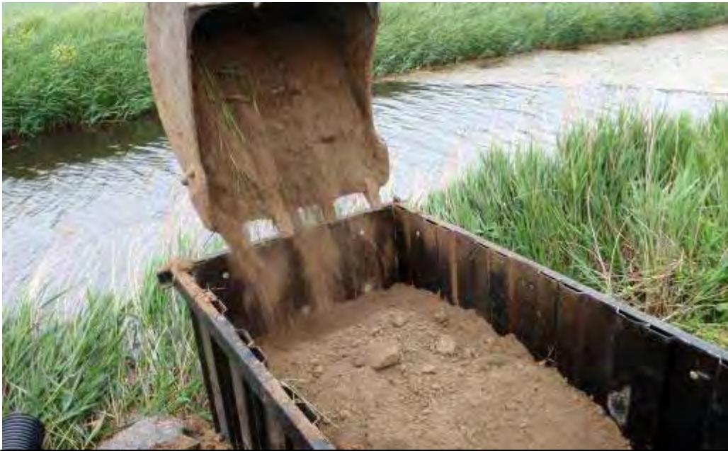
A stand-alone kingfisher nesting site in the process of construction at Ramsey First (Hollow) IDB as part of pump replacement mitigation works. Fine silt is used as fill for tunneling in the area behind the 50mm holes in the sheet piles on the drain side. This design also incorporates an otter holt below the kingfisher nesting level.
