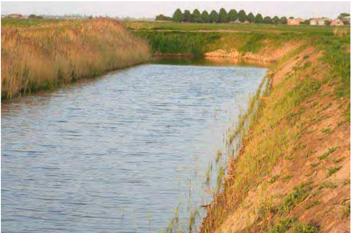
A re-profiled bank in March & Whittlesey IDB. The opposite bank was left un-mown for water voles to move to. A shelf was created at the toe and planted with sedge plugs.
