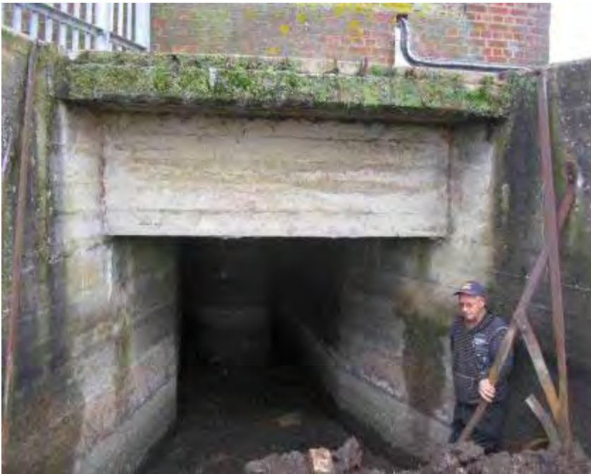
An old inlet chamber could provide a potential hibernation site for bats such as this one at Pidley Pumping Station, suggested by Bob Wilmer, District Officer, Warboys, Somersham and Pidley IDB.
