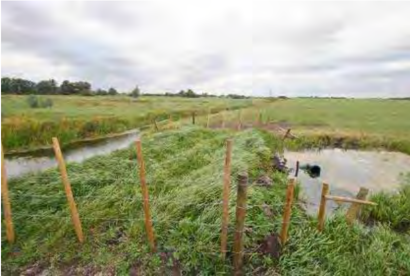
A twin-wall polyethylene pipe and turnable right-angled bend being used to control water levels in privately managed ditches of the Hundred Foot Washes IDB (the Ouse Washes).
