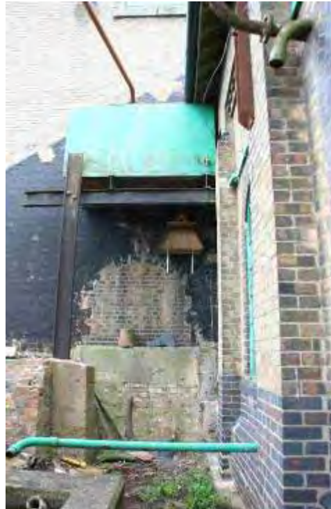
A well sheltered location under a redundant water tank proved a good site for this external box at Mepal Pumping Station.
